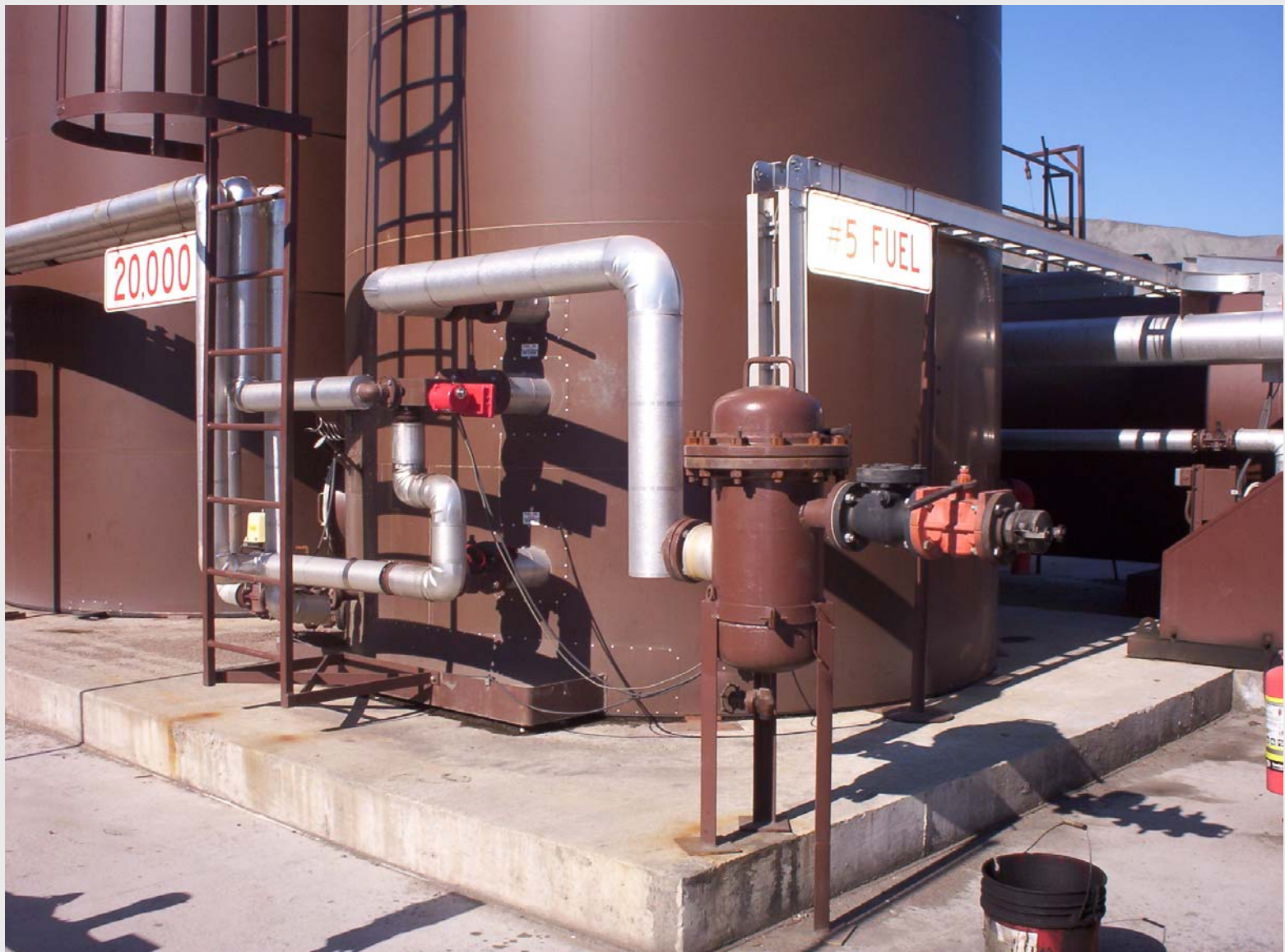
FILTER AT UNLOADING POINT.
